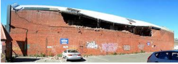
Figure 2: Out-of-plane wall failure caused by excessive diaphragm deformation [8].
