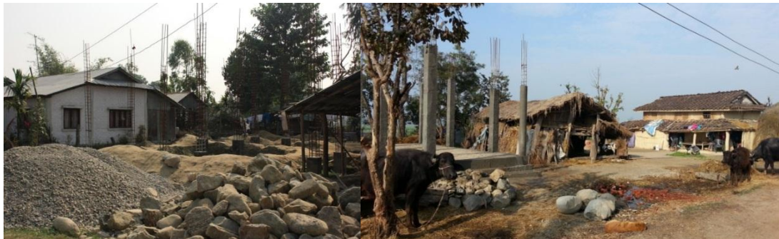
Plate 5.1 New building construction works employing reinforced concrete systems in Damak (left) and Dhangadhi (right).
