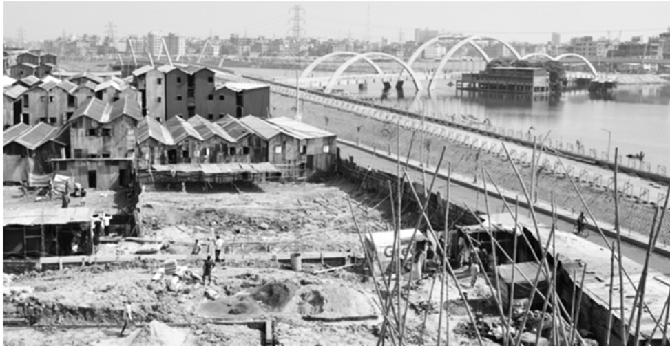
Figure 7-20: Hatirjheel area during the construction in 2011, eviction of informal housing (source: Prof. Dr. Shayer Ghafur)
