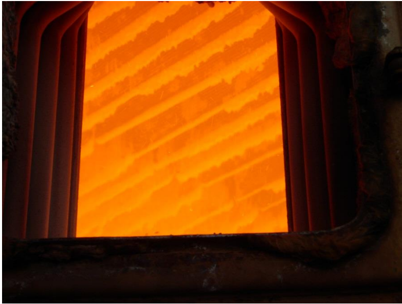
Figure 7. Slagging on the superheater tubes in a brown coal power station boilers.
