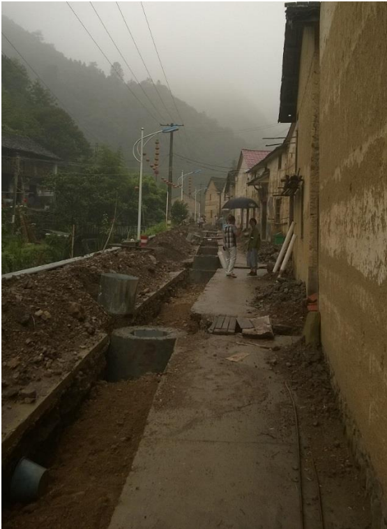
This is a different village, in the Dafan region, where they were also upgrading the sewerage system.
