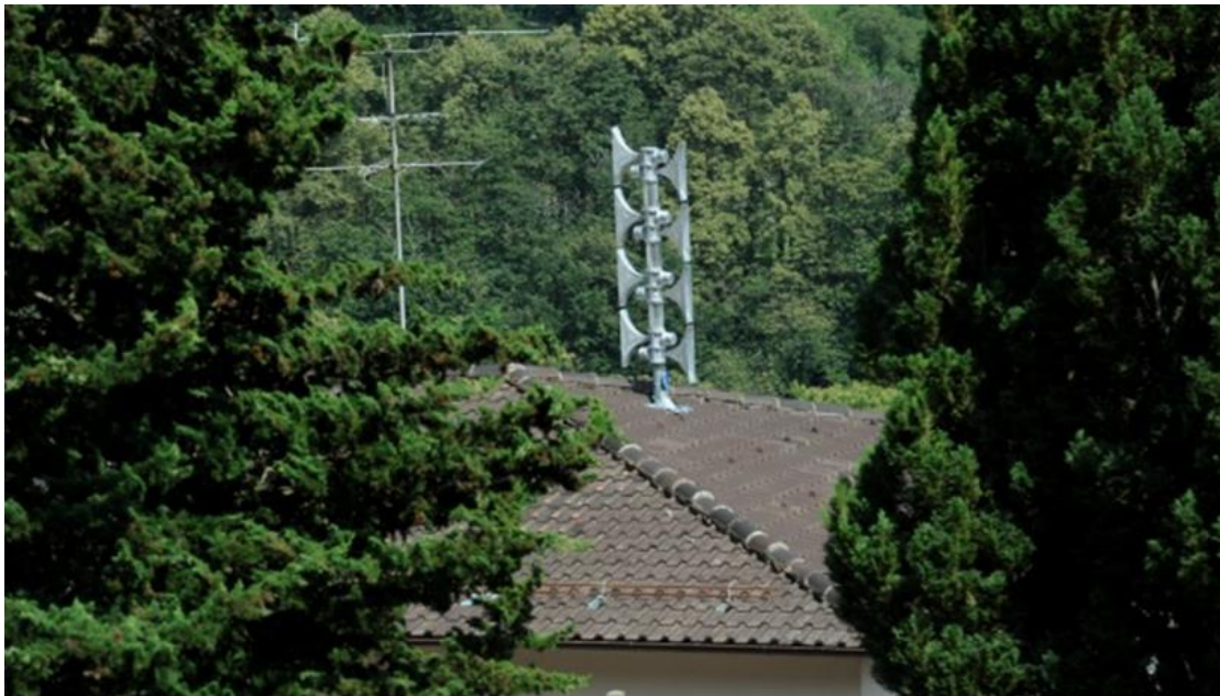
Plate 3.1: Emergency alert system across the nation, Swiss Polyalert sirens on house rooftop
