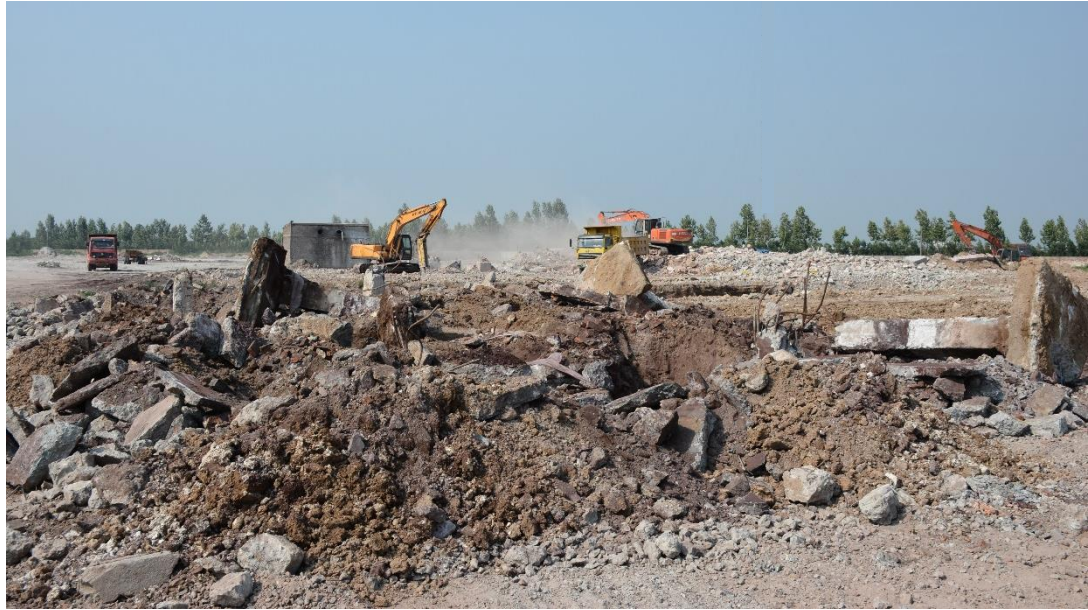
Figure 7.8 Demolition and removal work at the site, as of July 2017 (Source: author)
