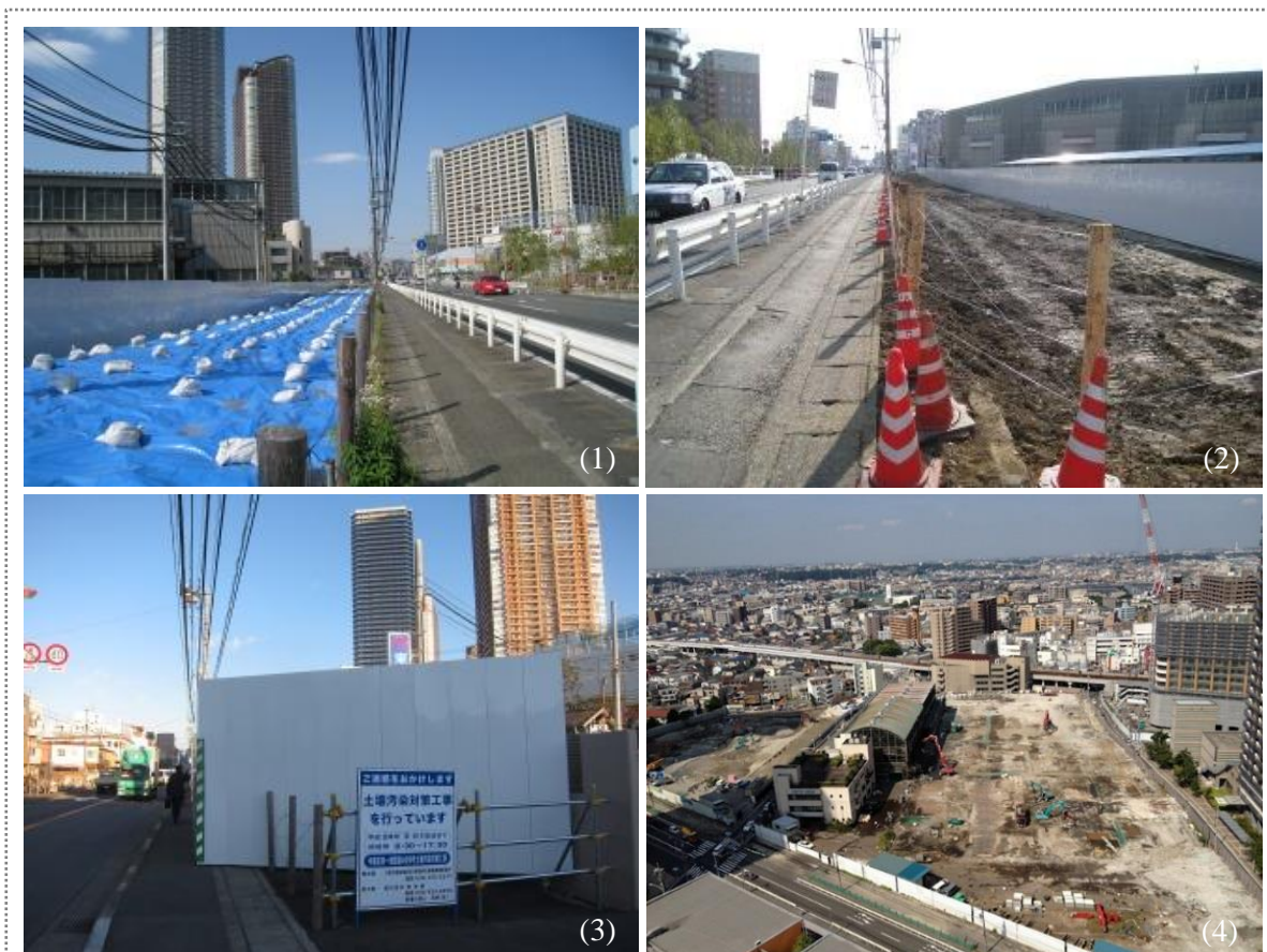
Figure 6.7 Soil remediation measures during the widening projects of Tsunashima (picture no. 1, 2) and Fuchu highways (picture no. 3), as well as the construction projects on the former site of the TKS factory (picture no. 4)
