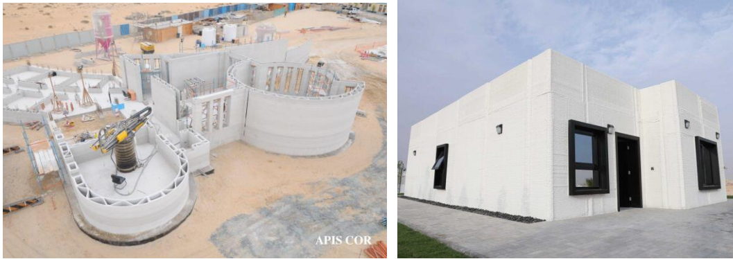
Figure 1. 3DP building in Dubai by Apis-cor (Left) (Apis-cor 2019), and 3DP house in Saudi Arabia by CyBe (Right) (CyBe 2019).
