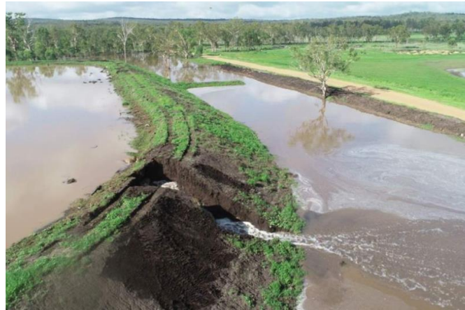
Figure 1.4. Talgai dam leak in Southern Queensland, Australia (Bavas et al., 2020)
