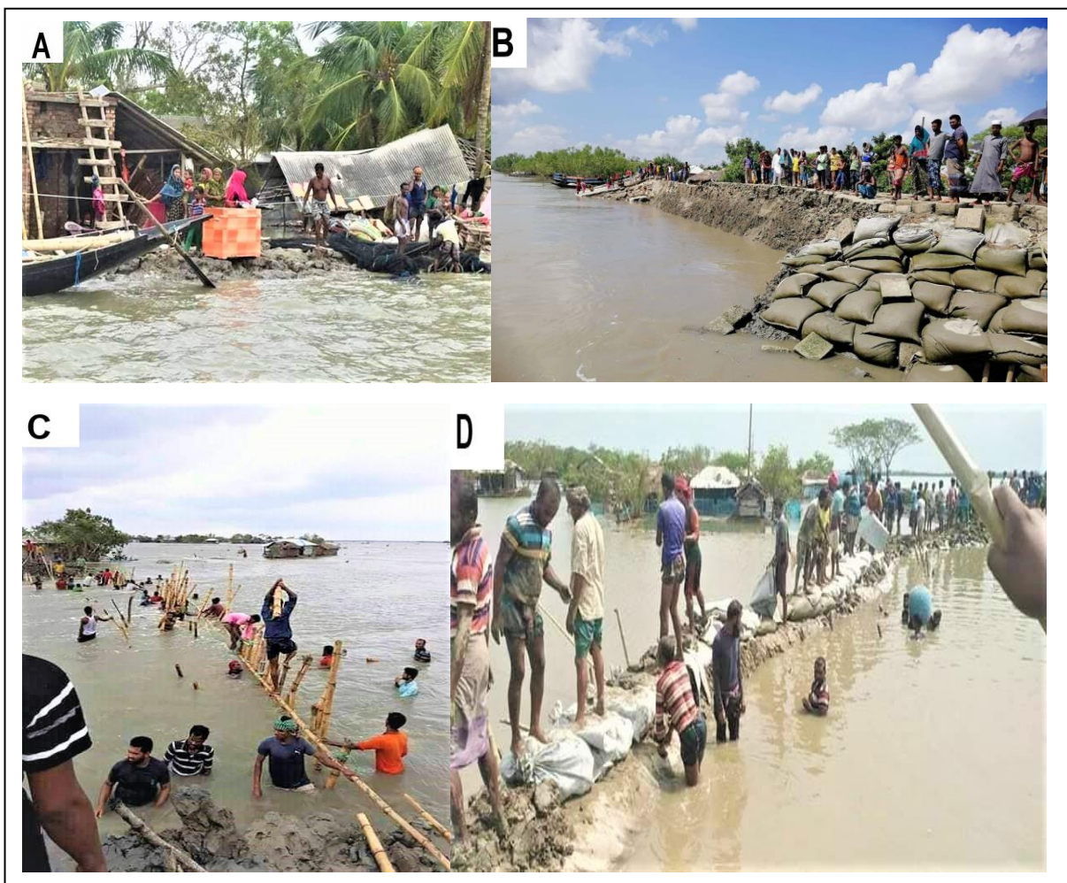
Plate 6.4 Males and females were engaged in repairing houses and a collapsed embankment in the cyclone-affected Gabura union.
