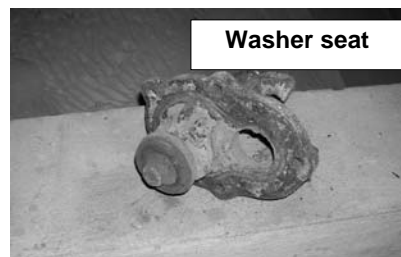
Figure T-1 – Details of the internal configuration of a fire plug/air valve as installed on the Hanson Transmission Pipeline
