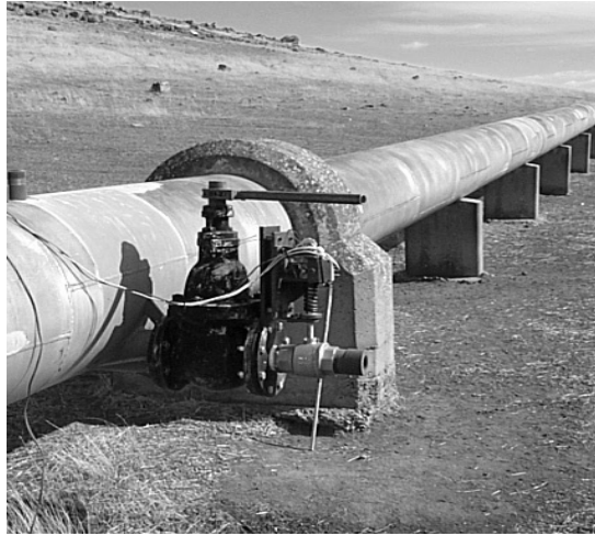
Figures N-1 - Typical collar ring restraints and saddle supports on the Hanson Transmission Pipeline
