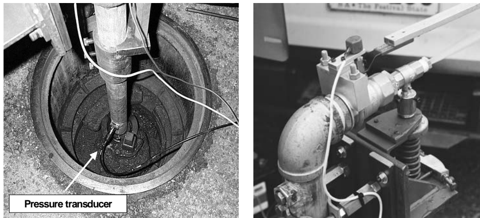
Figures 6-4, 6-5, 6-6 and 6-7 – Photographs of the transient generator as installed, bracing arrangement, base connection and valve/torsion spring arrangement
