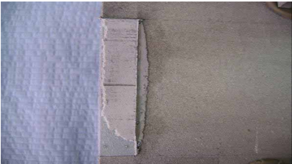
(b) Adhesive layer at failure
