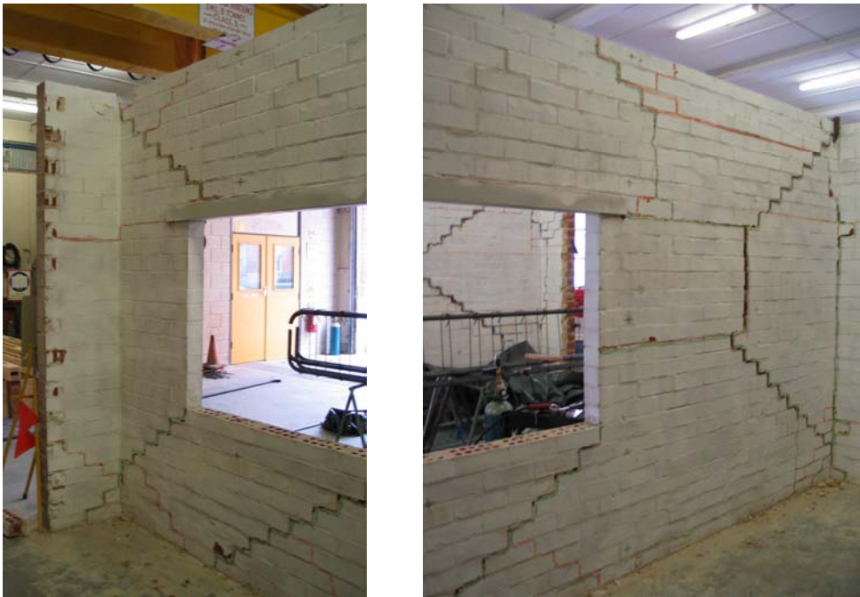
Figure B.36: Photograph of wall S5 crack pattern at the conclusion of cyclic testing.
