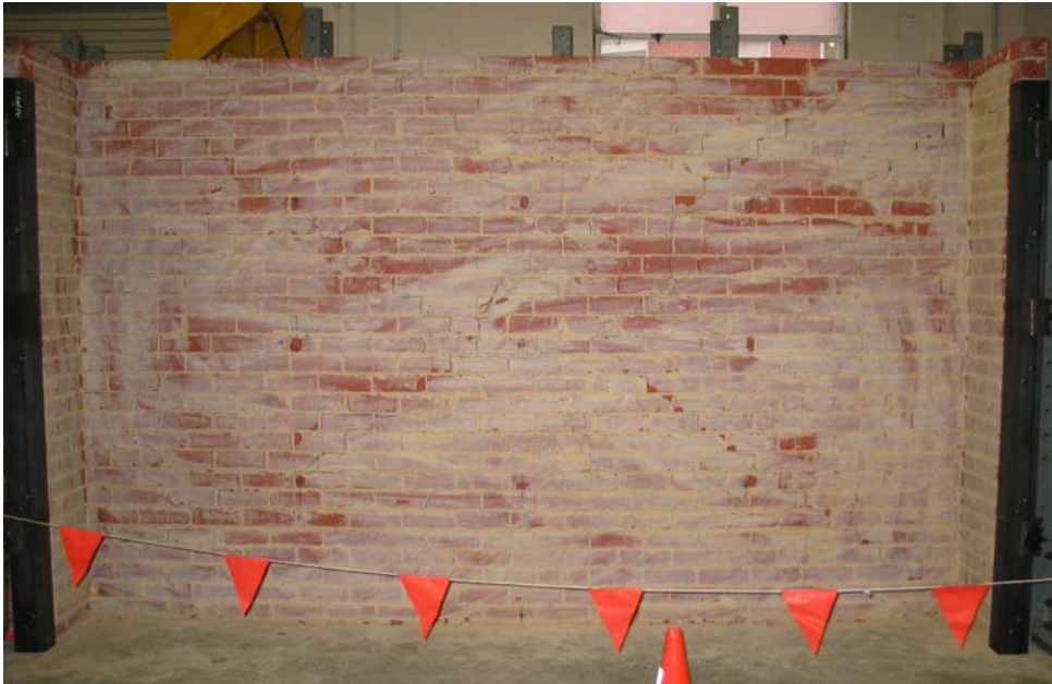
Figure B.32: Photograph of wall s1 crack pattern at the conclusion of cyclic testing.
