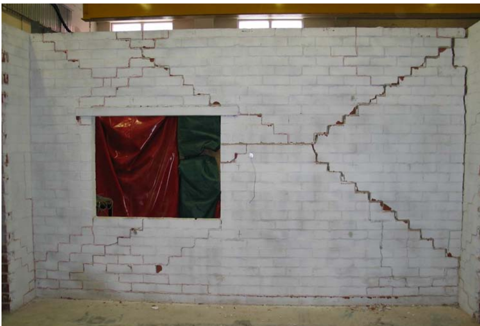
Figure B.35: Photograph of wall s4 crack pattern at the conclusion of cyclic testing.
