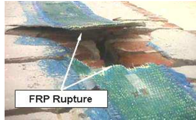
(c) FRP rupture
