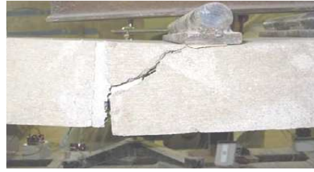
(b) FRP rupture
