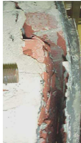
(e) Compressive Failure
