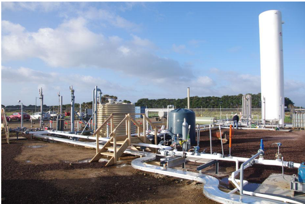
Fig. 1. The surface layout at the Otway Project site. The CRC-2 wellhead is left of centre, the CO 2 storage tank is at right and water pipes are in the foreground. The water storage tanks are out of the frame to the right.
