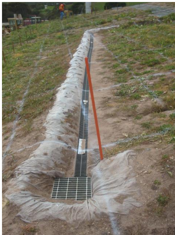
Figure 4.9 Runoff Collection Guttering and Drainage Check Pipe
