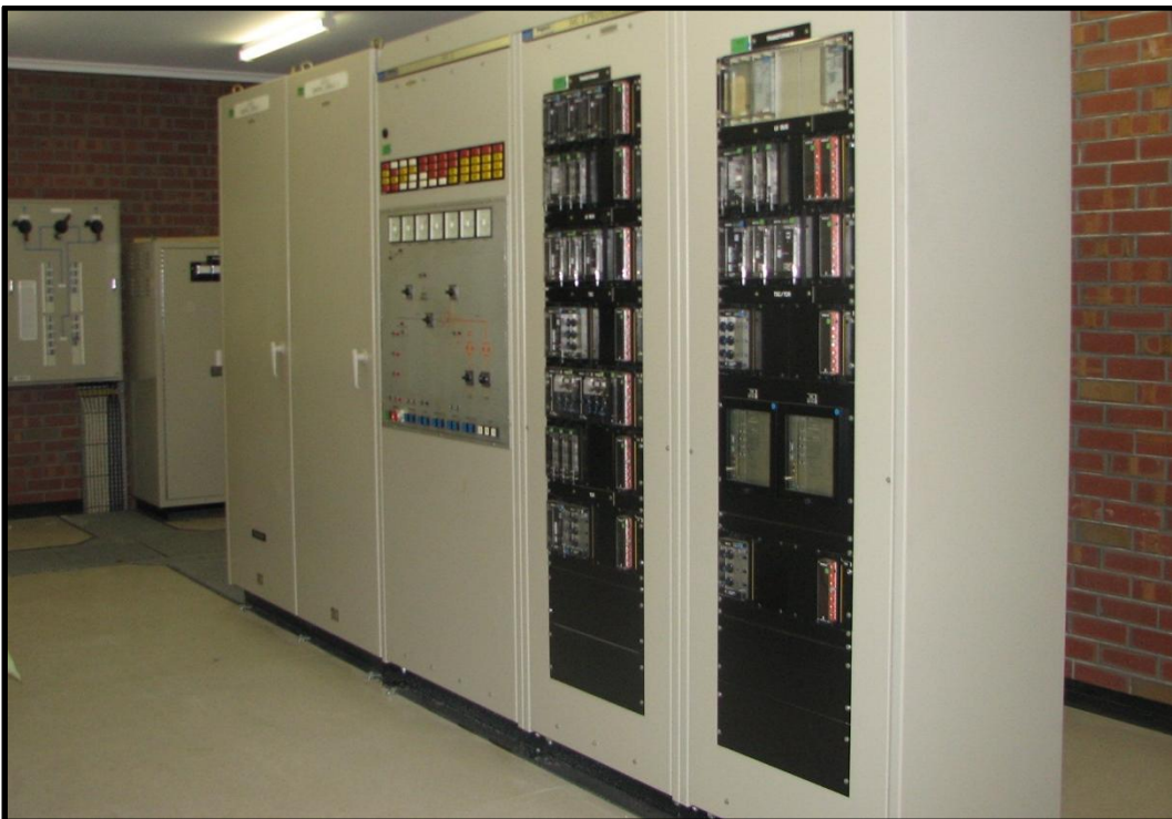
Figure 1.2: Substation automation system within control building
