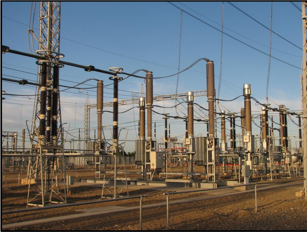
Figure 1.1: High voltage substation primary equipment at switchyard
